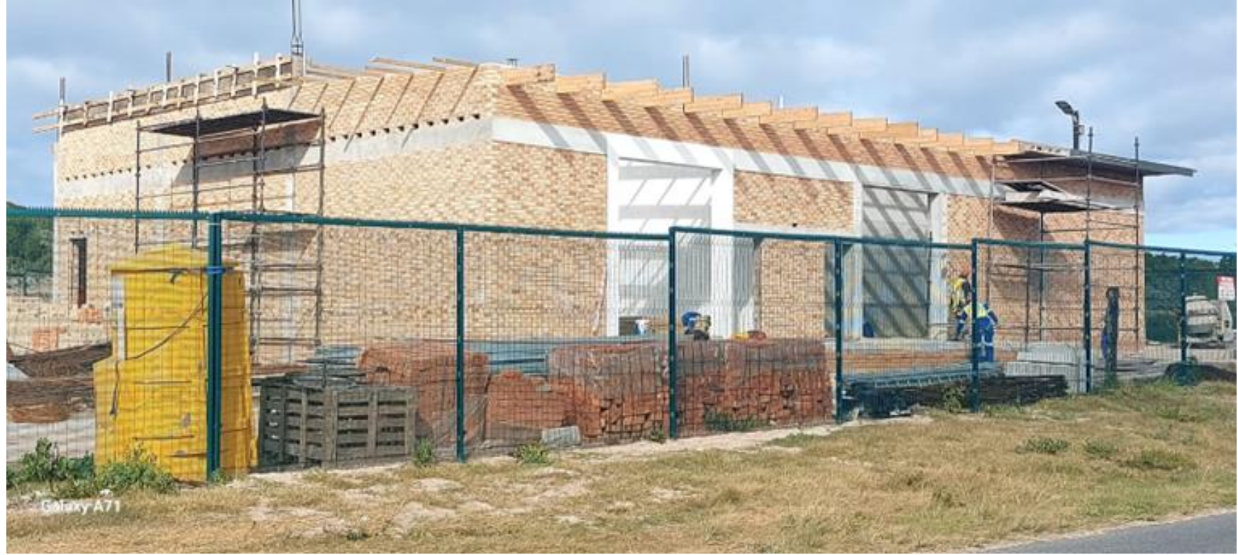
Birkenhead 66kV Substation and Overhead lines
